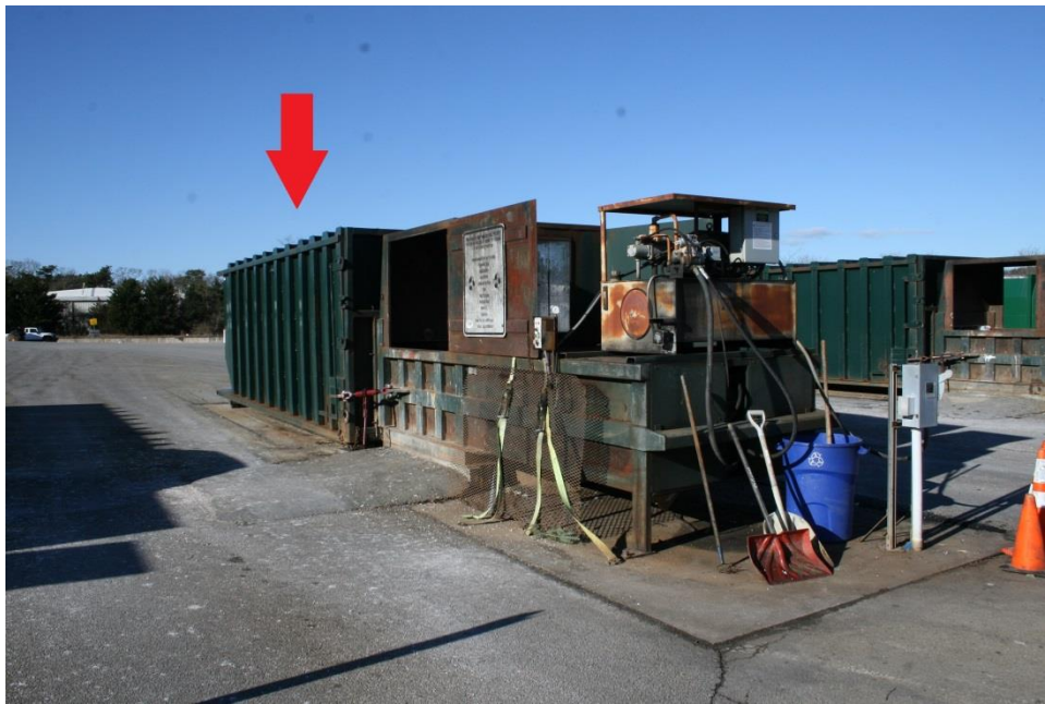
Containers with Corrosion
