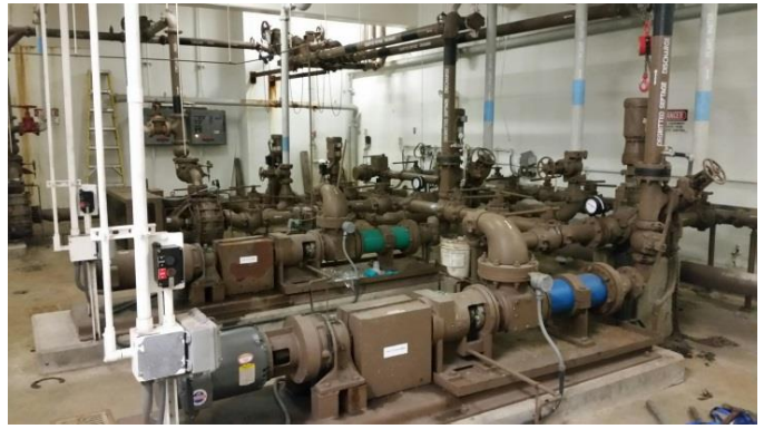
Sludge pump room
