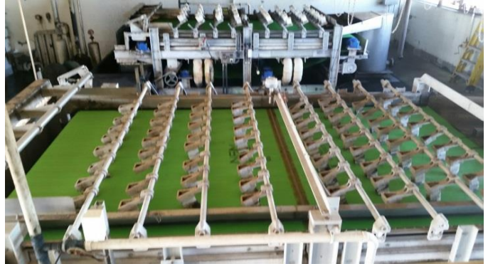
Sludge thickening belt
