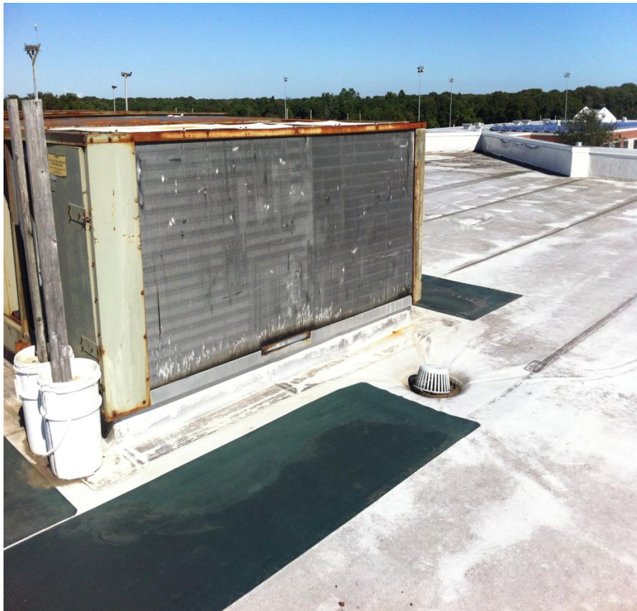
Roof Top ventilators
