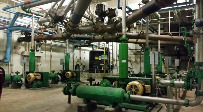
Septage Blower Room
