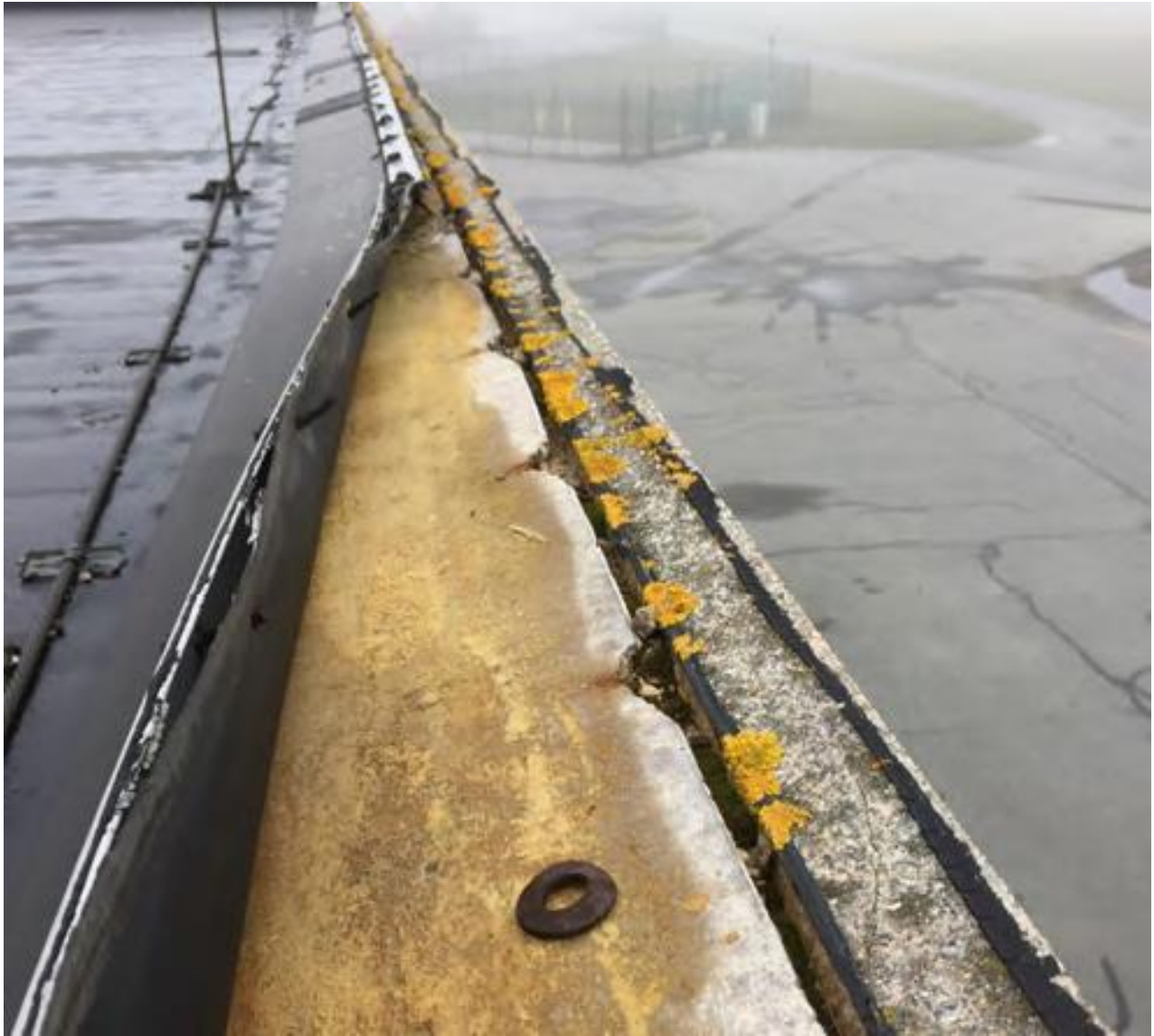
Roof Repair Needed
