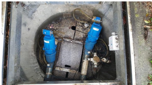
Vacuum Sewer Valve Pit
