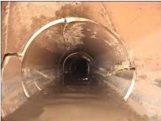
Defects in Pipe (Not a Barnstable photo)
