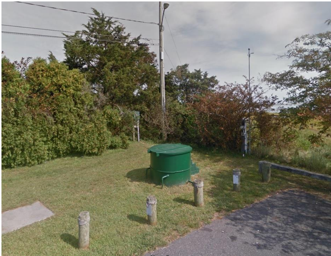
Rendezvous Lane Pump Station
