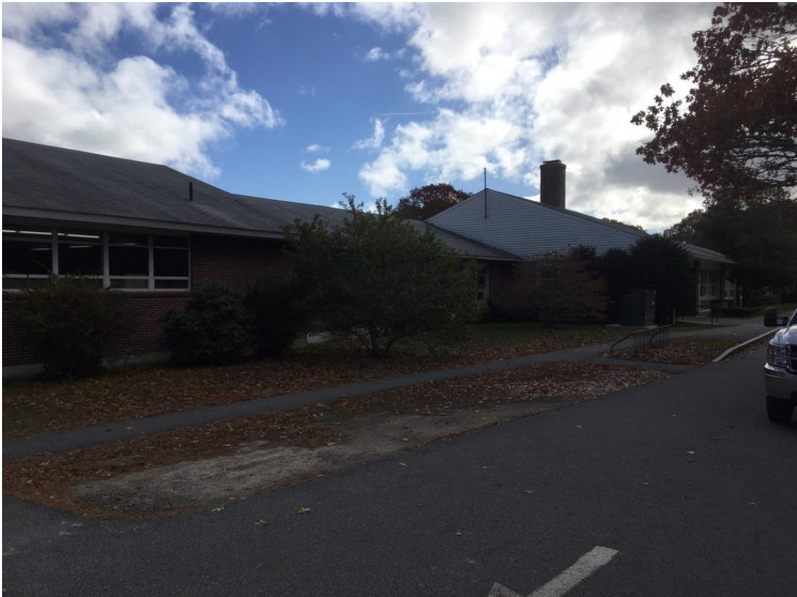
Centerville Elementary School Needs Roof Replacement
