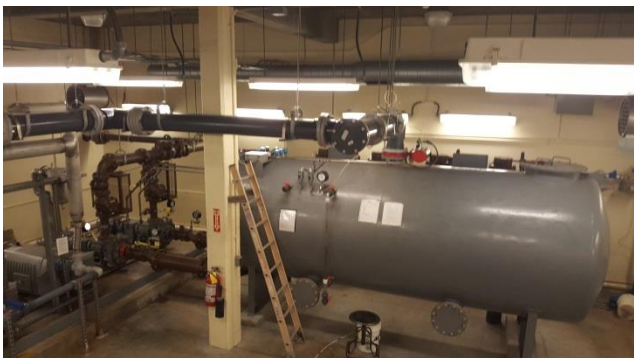
Vacuum Sewer Collection Tank
