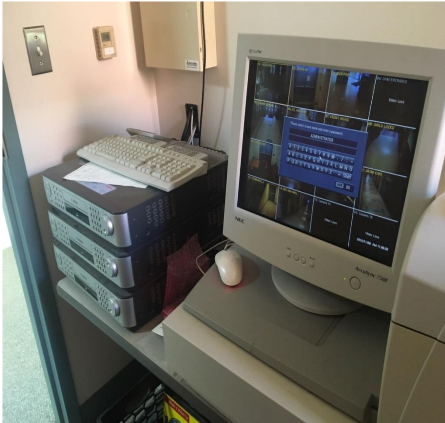
Typical Surveillance System
