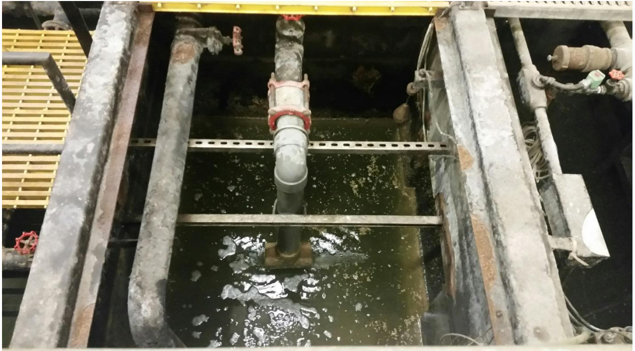
Denitrification Sand Filter Tank
