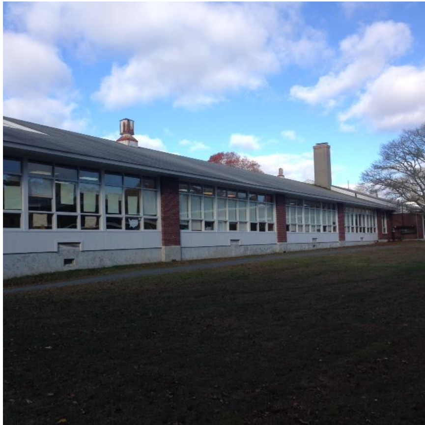
Centerville Windows Need Replacing
