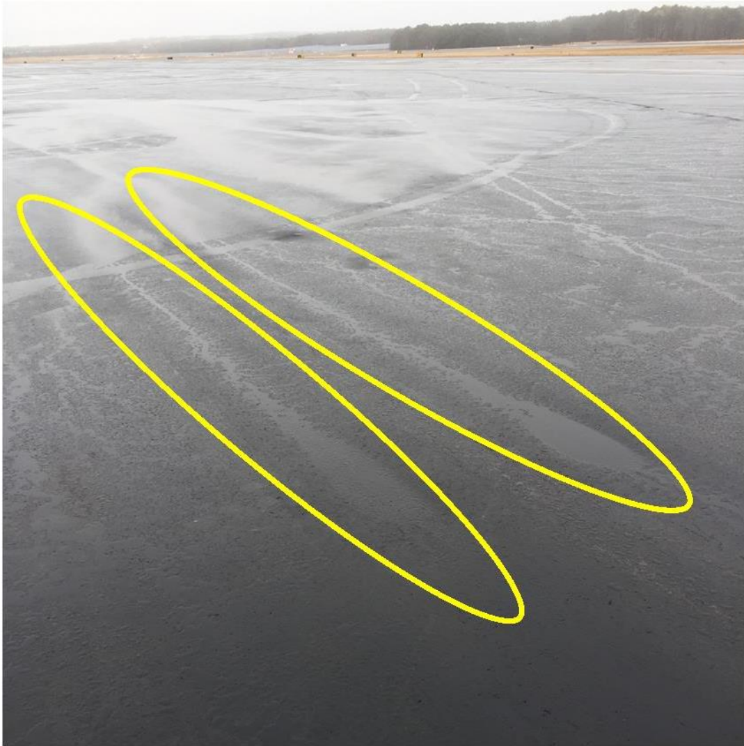
Pavement Depressions due to Heavy Aircrafts
