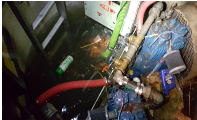
January 4 Station Flooding
