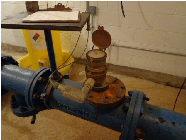
Examples of Pumps and Valves
